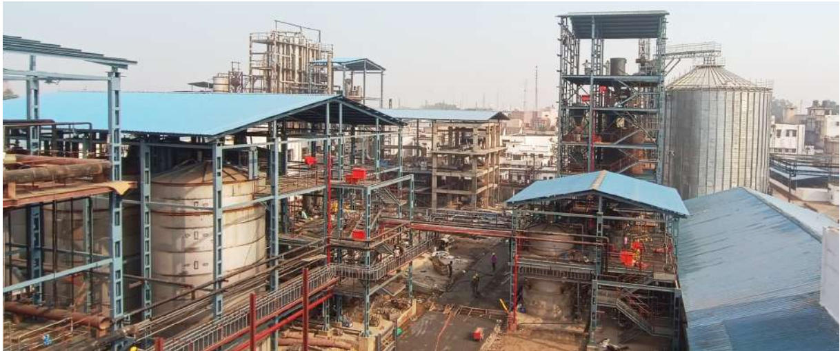
Aerial view of Grain Distillery - Expansion of Modi Distillery, Modinagar The commercial production has started from March 2024.
